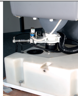
waste water tank and technics
